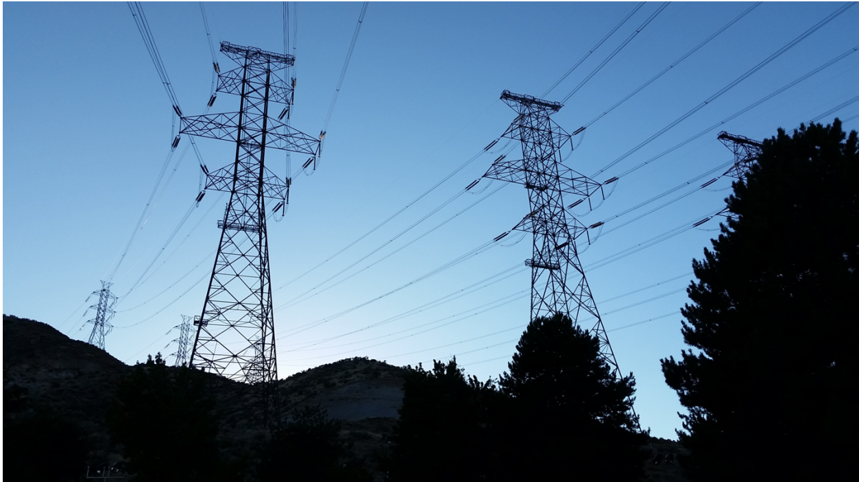
Figure 10. 500 kV Three-Phase Electric Power Transmission Lines
