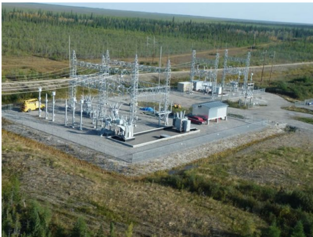
Figure 15. Kashechewan Sub Station
